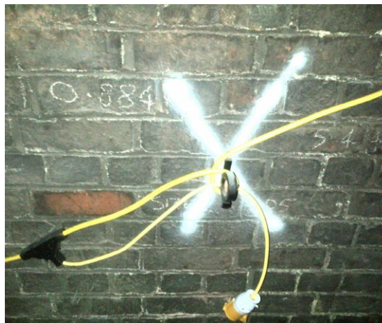
Image shows a 110v cable being looped over a piece of equipment – this is an example of incorrect use
