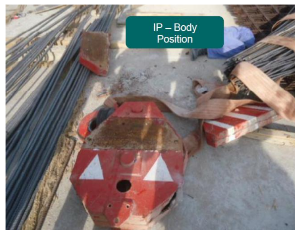
Image shows the failed hoist and fallen the load
