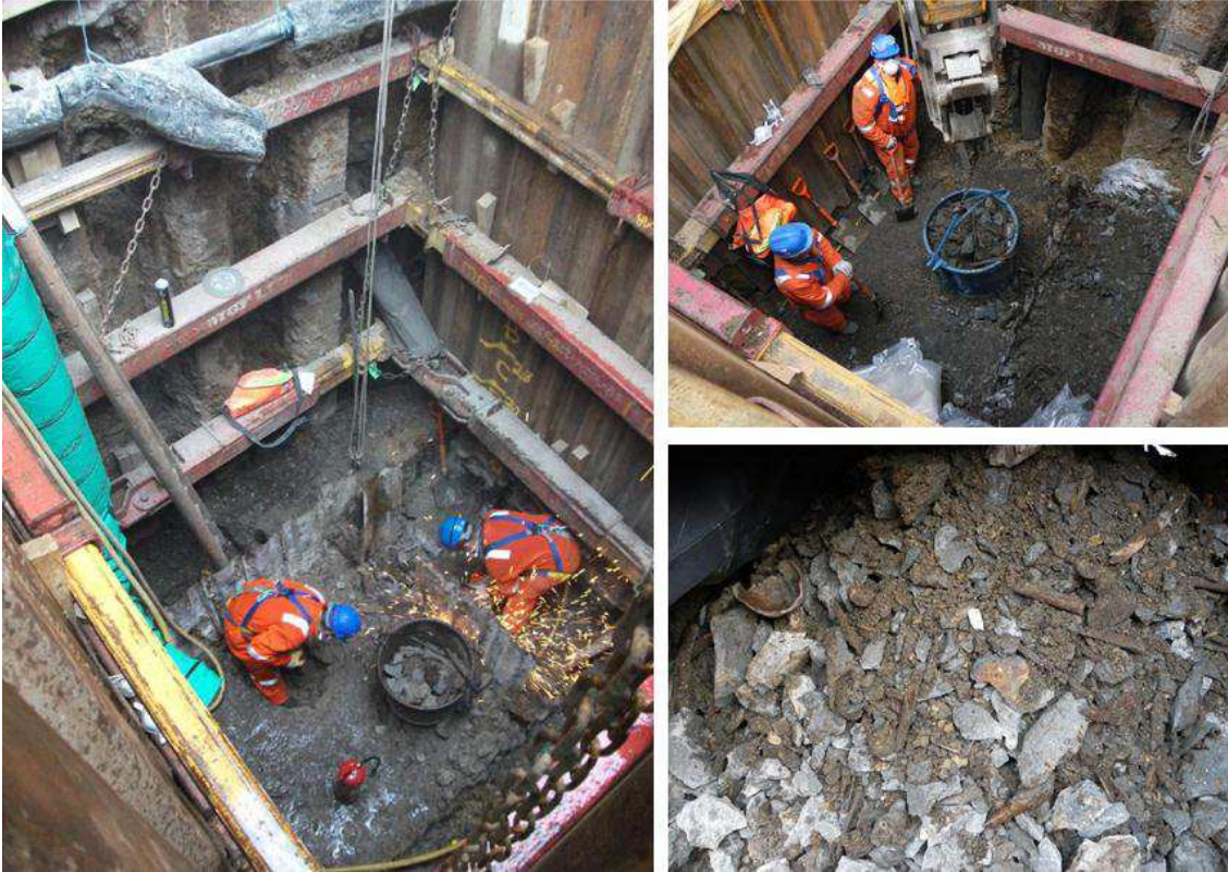
Fig. 16 – Excavation of 1985 reburial site. Below right: Fragmentation of remains that were reburied mixed with concrete (Copyright: Crossrail)
