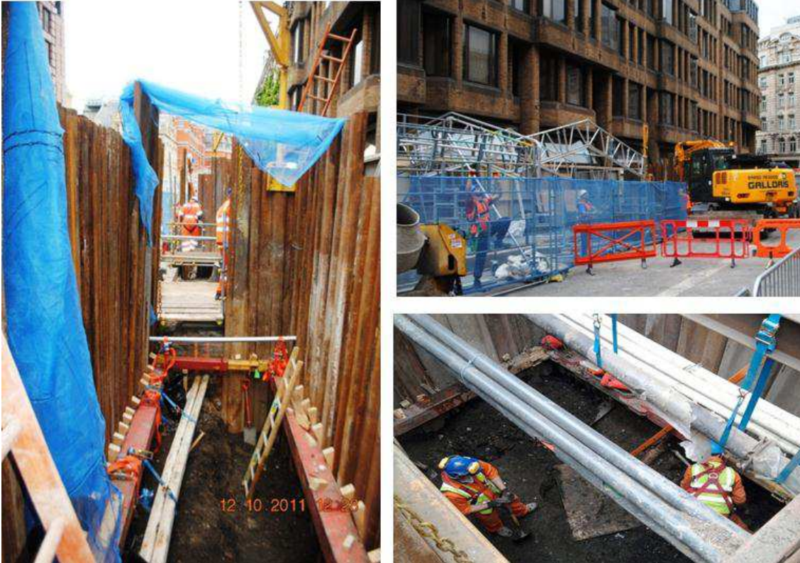
Fig. 13 – Liverpool Street exhumation in progress for south pile line (Copyright: Crossrail Ltd)
