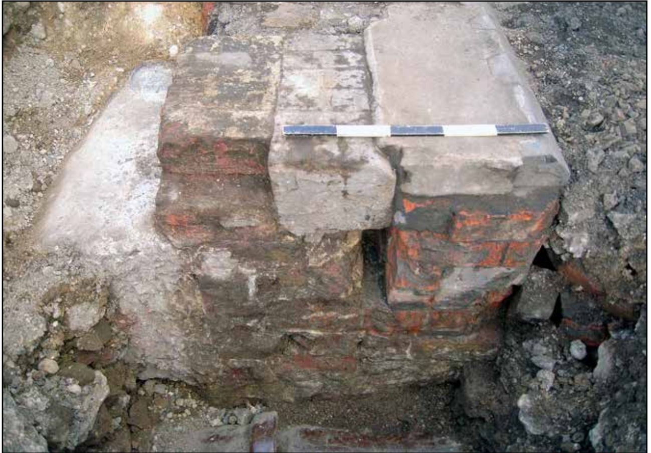
Plate 51: Section through inspection pit sidewalls the southern wall of broad gauge pit on southern sidewall of standard gauge pit
