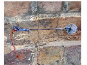
Vibrating Wire Crackmeter:
