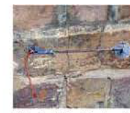
Vibrating Wire Crackmeter:
