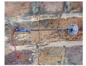
Vibrating Wire Crackmeter:
