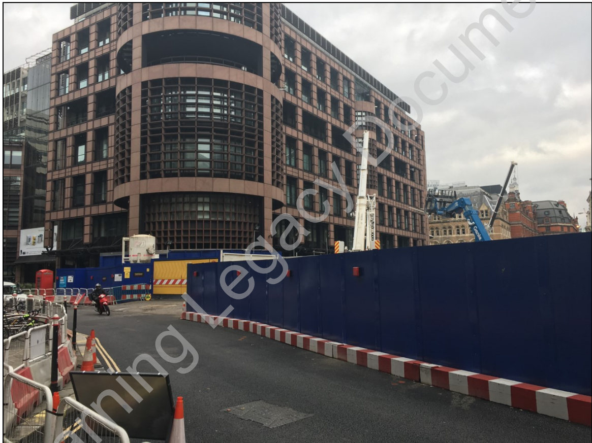
Figure 3 – C502 Site Obstruction
