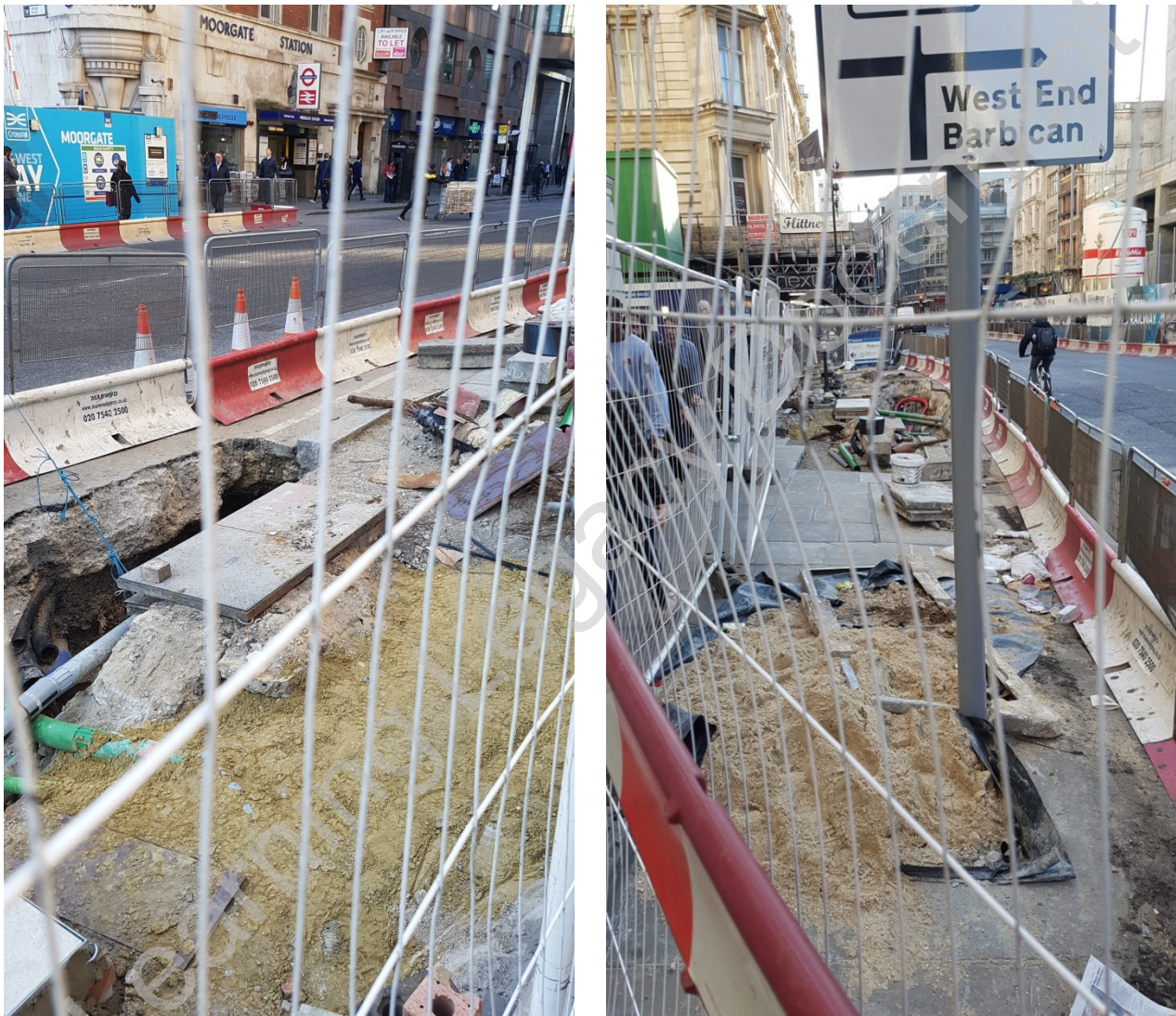
Figure 4. Roadworks taking place on Moorgate footpath. LP12347 to LP12355 affected by works.
