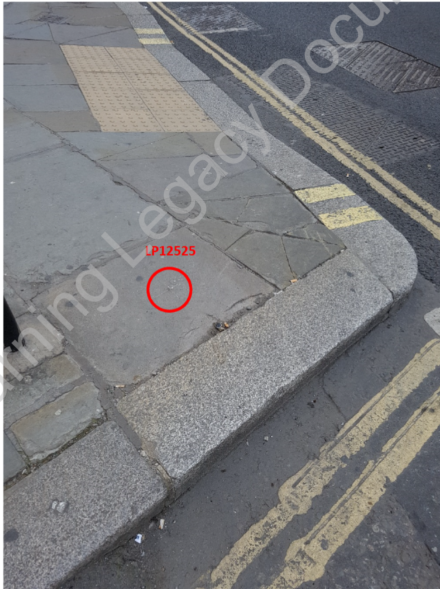
Figure 3. LP12525 Located on Unstable Concrete Slab
