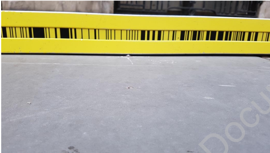
Figure 8. LP12437 Uneven slabs
