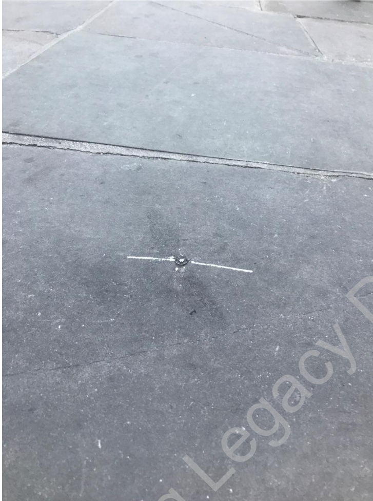
Figure 10. LP12455 Stud is damaged
